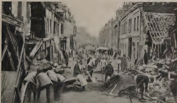
French engineers repairing the havoc in the Rue de Paris caused by retreating Germans. When they evacuated Noyon they mined the streets and afterwards heavily bombarded the town.
